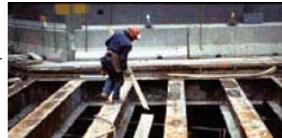
This worker is not protected by any of the protective systems that are required by OSHA.
